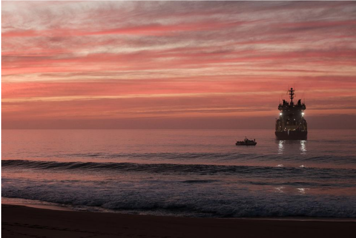
(Cable landing operation, European Commission, n.d.e.)
